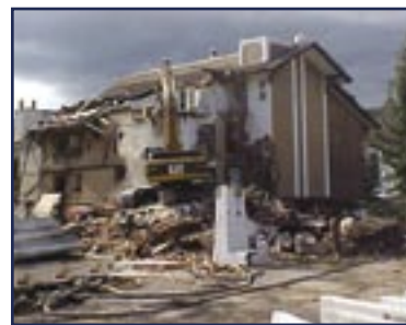
Demolition of the Swiss Hotel began in September, clearing the site for One Willow Bridge Road construction, currently underway.
